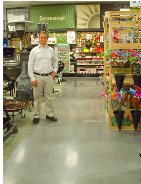
Contractor Nathan Christner was able to finish the floor using the HardWear method in cold temperatures where epoxy would not have cured, saving major expense by not needing to heat the building during construction.
